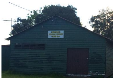
Pigeon Club building. Aged facility needing refurbishment
