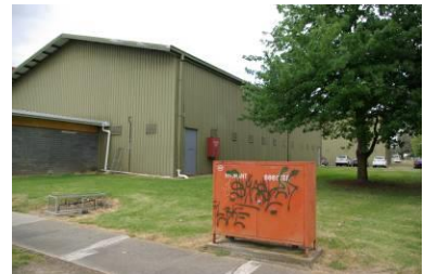
External fire services 'may' require upgrading as part of any sports reserve redevelopment.
