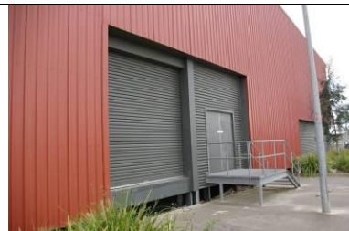
Loading bay – no protection to car parking light tower if vehicle is reversing.
