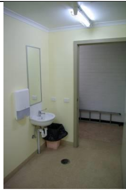
Accessible amenity – not complaint to current BCA / DDA requirements. Mirror not angled, no shelf unit and basin within door landing circulation.
