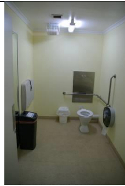
Accessible amenity – not complaint to current BCA / DDA requirements. No backrest to pan.
