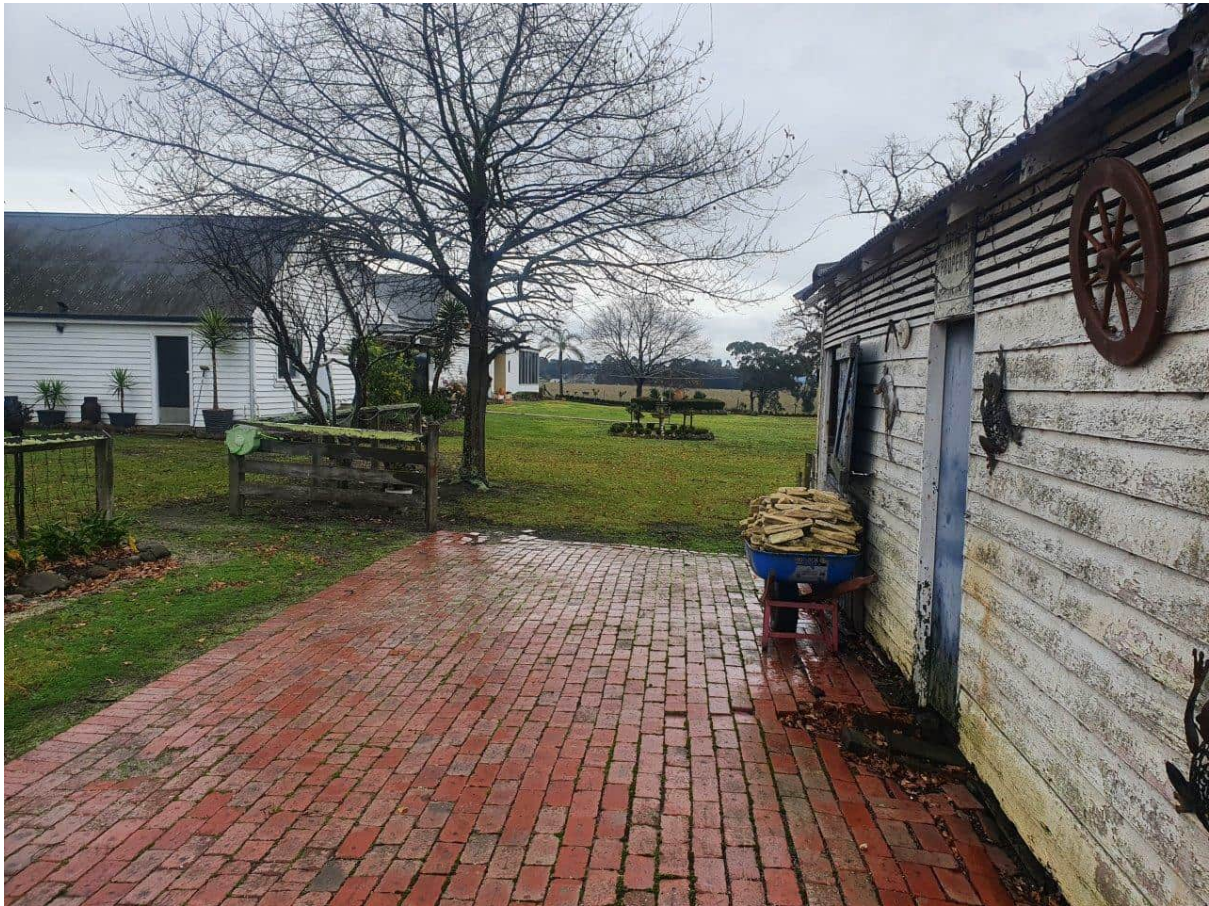
Photograph 3: View of a small shed in the homestead area. Potential lead paint was observed on the shed exterior. The main residence appeared to be painted with non-lead paint.
