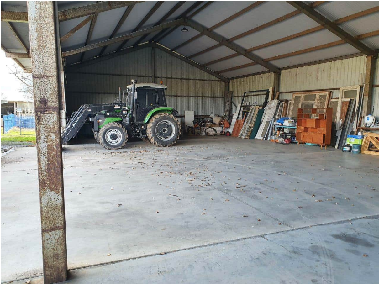
Photograph 1: View of the large shed in the homestead area onsite. The concrete floor appeared to be in good condition.
