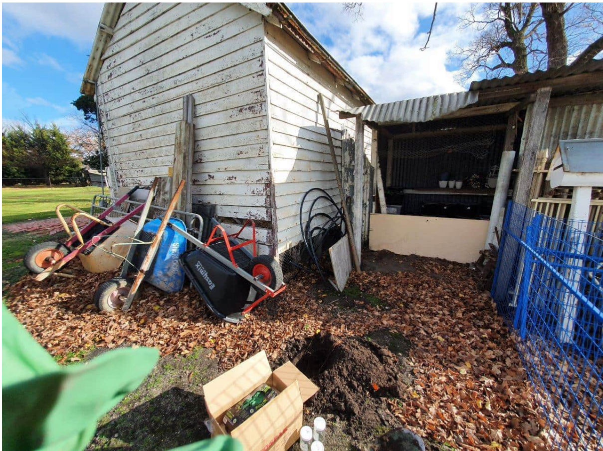
Photograph 2: View of a small shed in the homestead area. Potential lead paint was observed on the shed exterior.
