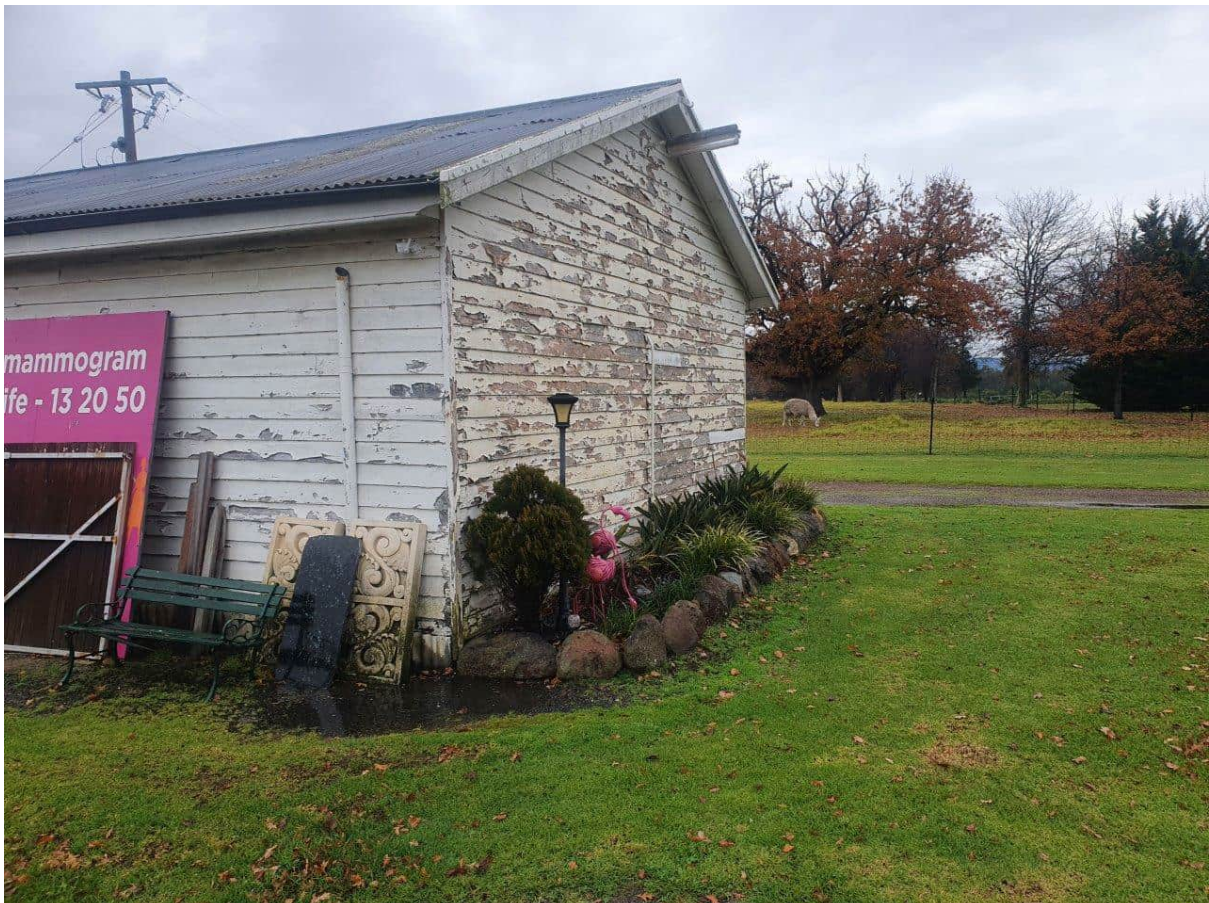
Photograph 6: View of another small shed in the homestead area onsite. Potential lead paint was observed on the shed exterior.
