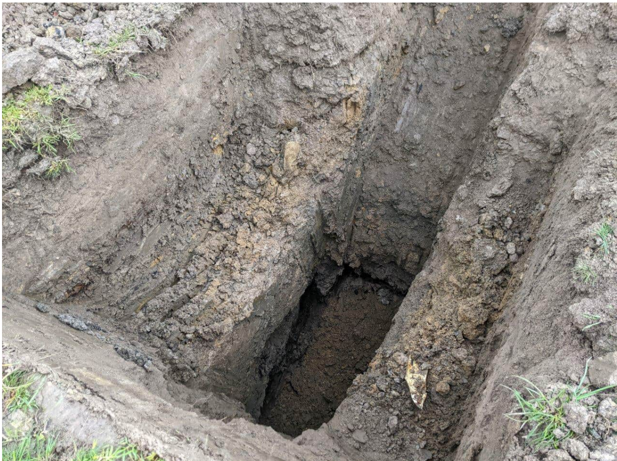
Photograph 16: View of TP01. Trace fill inclusions were observed within test pits within the filled area.
